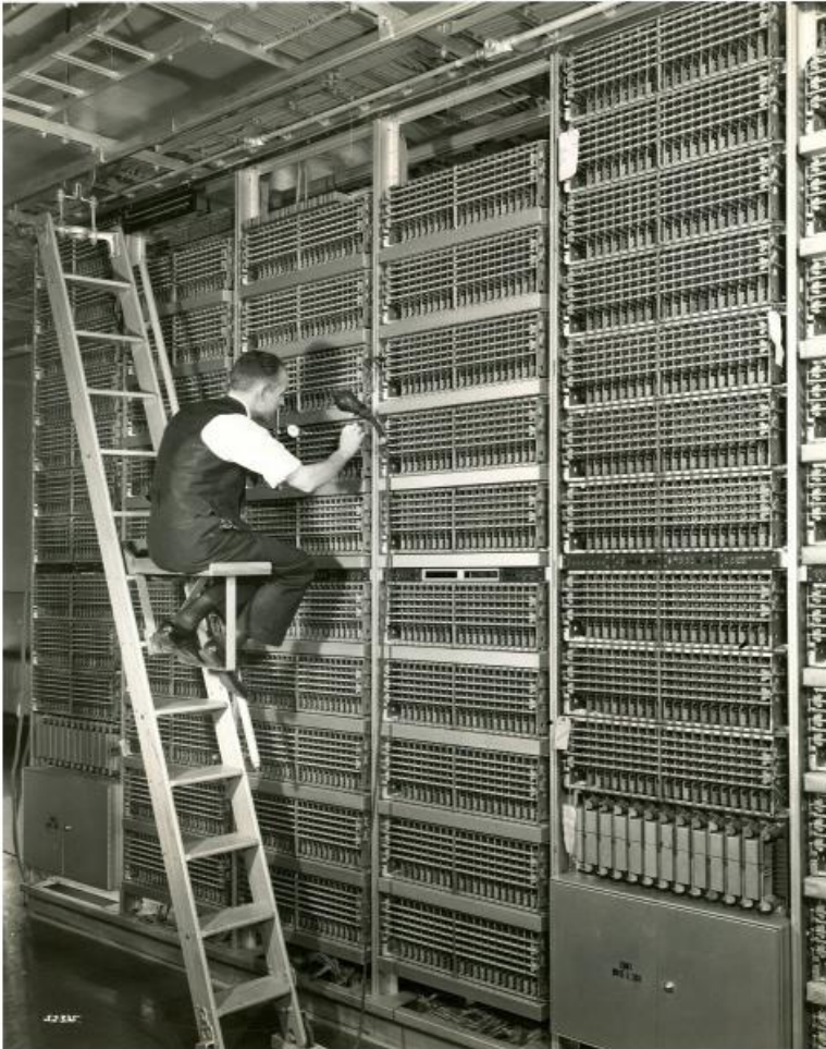
#1 crossbar switch, East 30th St., New York, New York, 1938.
